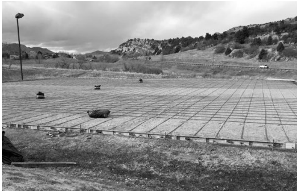
This photo shows the tension cables before the court surface was poured in mid-March.
