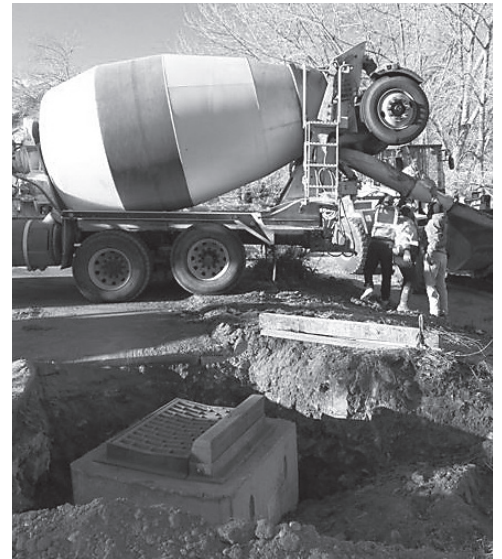
Parking lot drain line inlet. Wet concrete was transported by a front loader to where it was poured and finished.
