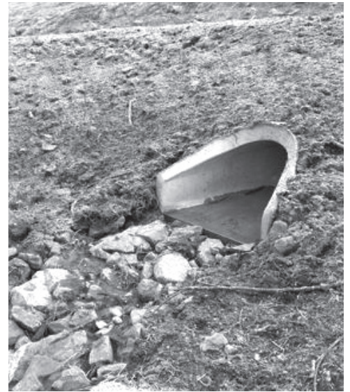
Outlet for eastern drain line.
