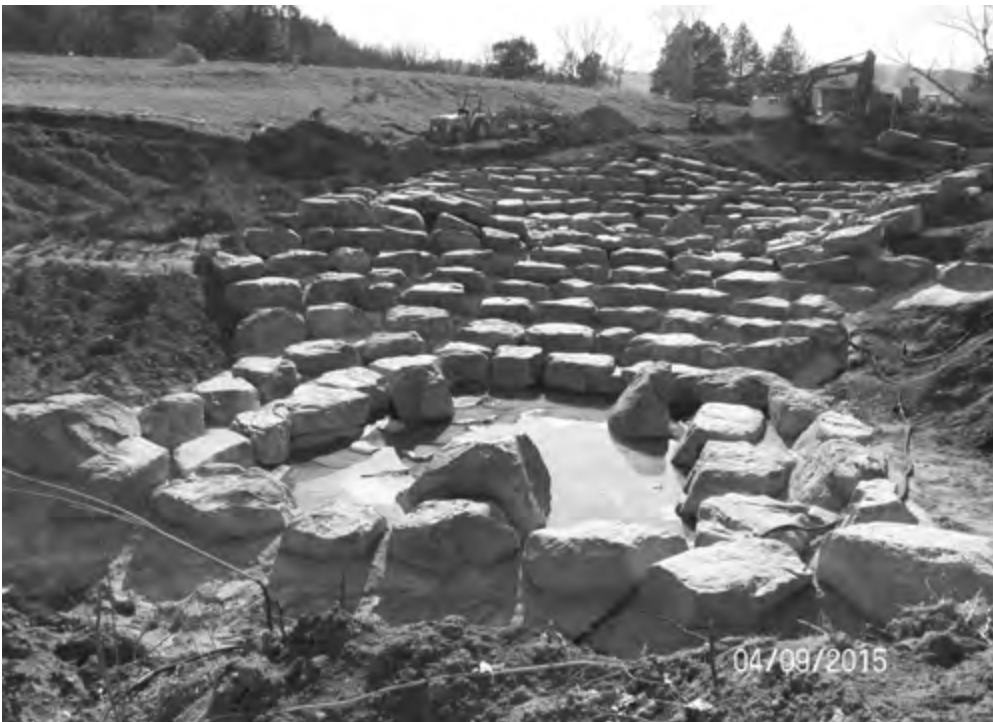
View from downstream end of project showing first two completed, grouted, boulder drop structures. The project is about 50 percent complete and will wrap up late summer 2015. In addition to stabilizing the stream channel, the project will create a natural surface trail link, along the north side of the site, to Brannon Gearhart Park, and there will be a new sidewalk along Club Drive connecting to South Valley Road.
