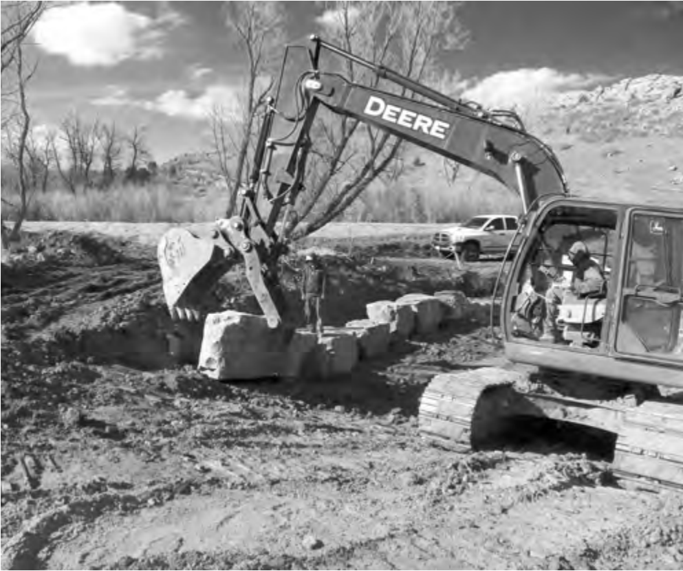
The Massey Draw Stream Stabilization contractor, AGE, Inc., sets large boulders as construction on the third and final grouted boulder drop structure continues. The structures will stabilize erosion, address public safety hazards associated with the site by the Community Center, improve water quality and protect wetlands. The total project cost is around $460,000 and is paid for entirely by Master Association dues.
