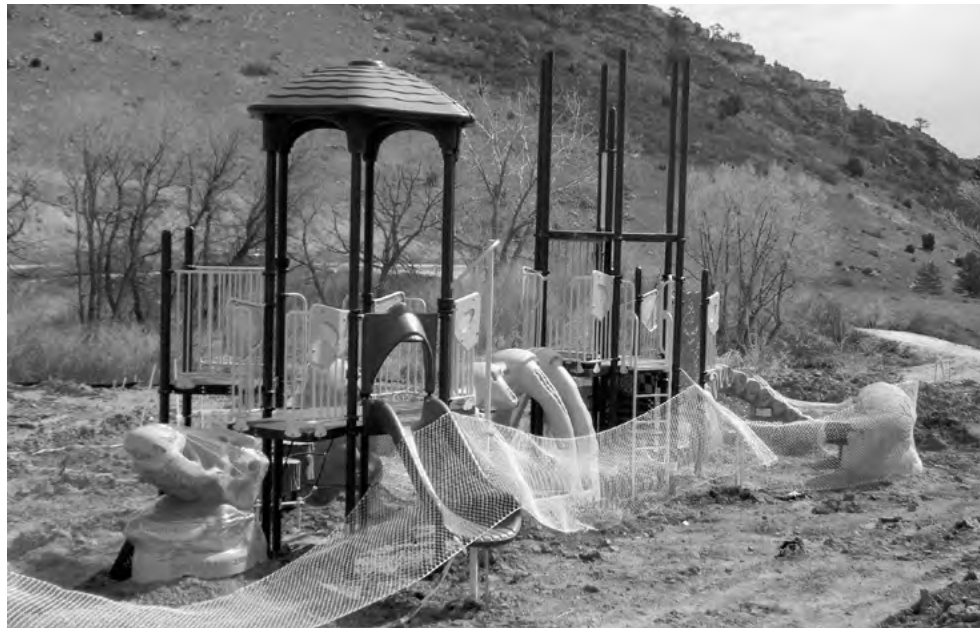
The new dinosaur-themed playground on the east side of the Community Center is underway and is anticipated to open Memorial Day weekend.
