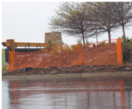
Damage to Rock Wall at Entrance to the Valley
