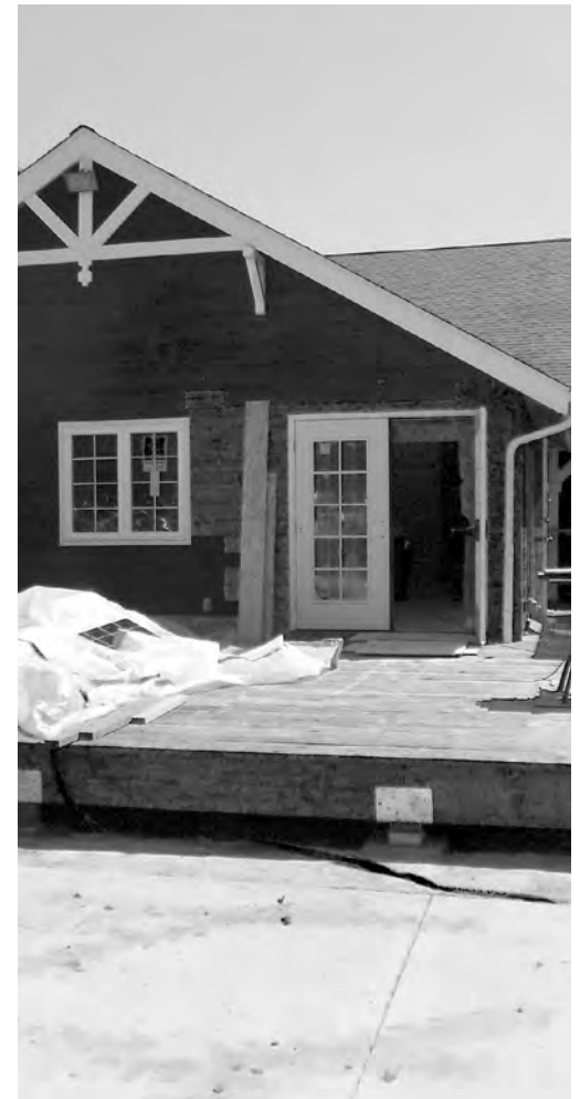
A new entrance is being added to the Recreation area on the south end of the Ranch House. The entrance features a concrete pathway leading from the parking lot to a new wooden deck and French doors. This new entrance is anticipated to open in late June, barring any weather or construction delays.
