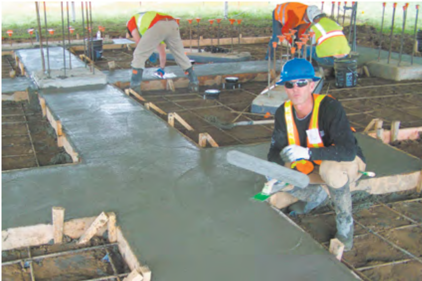
Ken-Caryl Ranch resident Chris Sullivan secured donations and contributions for material and labor for 100 percent of the concrete work on the Veterans Monument at Ken-Caryl Ranch.
