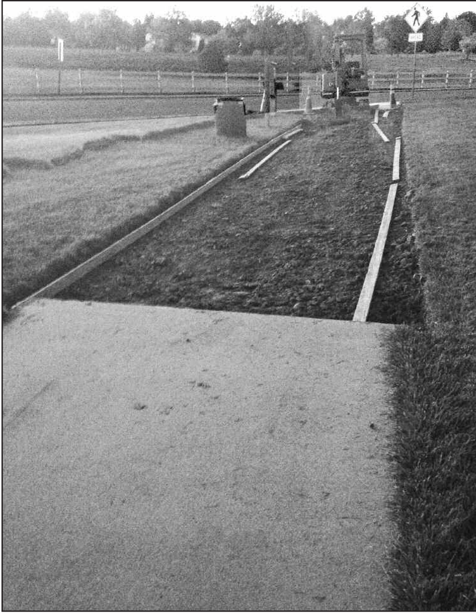
The Metropolitan District budgets money each year for concrete sidewalk repairs in parks throughout the community. The most recent repair was in Community Park, across the street from Shaffer Elementary.
