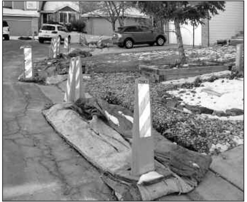
Thanks to Deer Creek resident Peter Wolberg for capturing this photo. Some streets in the Deer Creek neighborhood are getting new concrete gutters to replace the current, damaged gutters. The company doing the work is Concrete Express, Inc., and the project is being funded by Jefferson County. Along with gutter work, several streets will be repaved next year. We will be publishing the proposed schedule of paving work in a future issue of Life at Ken-Caryl.
