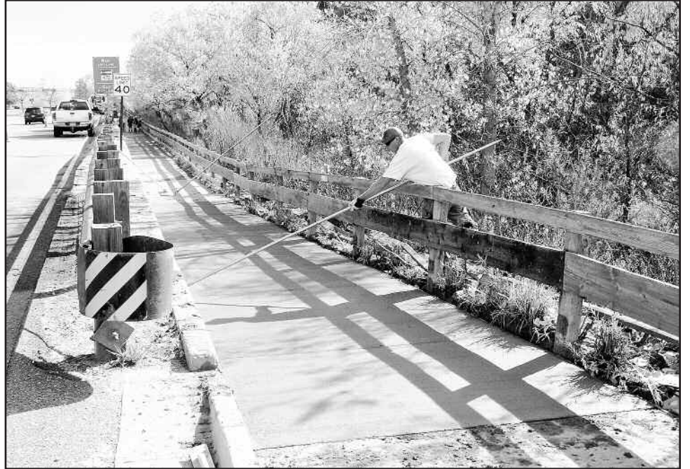
Work is now completed on the concrete path next to the entrance to the Valley. AGE Construction poured new concrete in late October, and the path is open for use!
