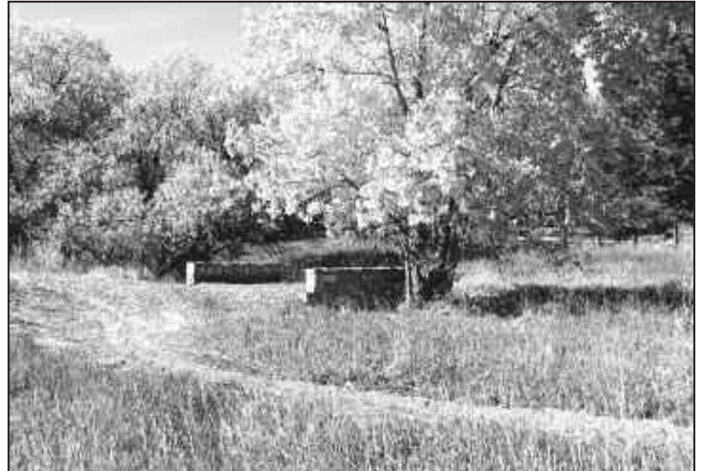
The Stone Bridge Trail is located north of Bradford Intermediate School and provides access to this newly-restored, historic, masonry bridge.
