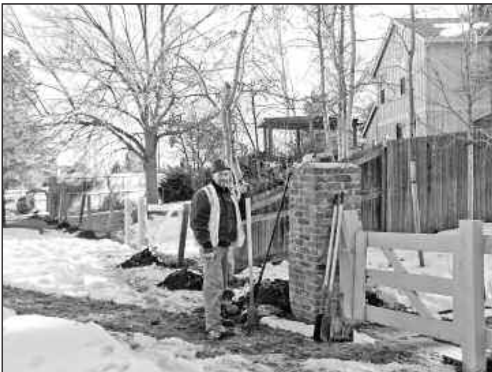
The Split Rail Fence Company is installing a new split rail fence along the south side Greenbelt E between Continental Divide Road and Chatfield Ave. The project will be completed by the end of March. The total cost of $23,746 is being paid by the Master Association.
