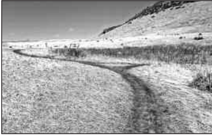
The Trail Club helped re-route the east portion of the Lark Bunting Trail. The re-route corrected significant erosion problems and detoured around sensitive habitat the old trail went through.
