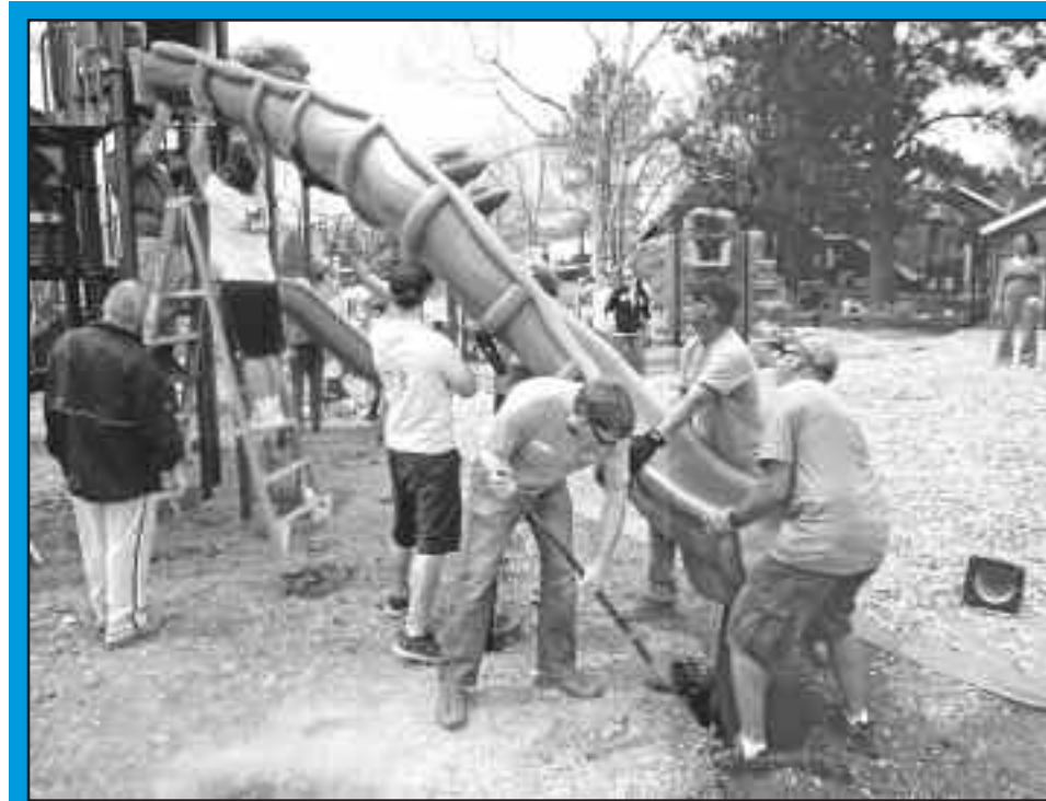
What a great community we live in! More than 100 volunteers turned out for the Ranch House Playground Community Build event on April 12. Thank you to everyone who helped! The new playground is now open and ready for kids. Check out the photos of the Community Build event on Page 9.
