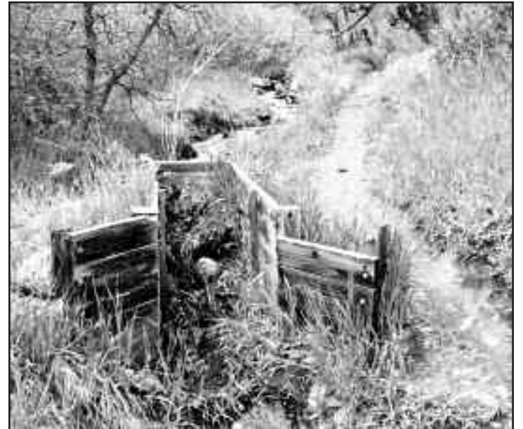
Don Ebner took this photo in 1999 of the same wooden structure on Massey Draw Trail. You can see by comparing the two photos that the structure is deteriorating.
