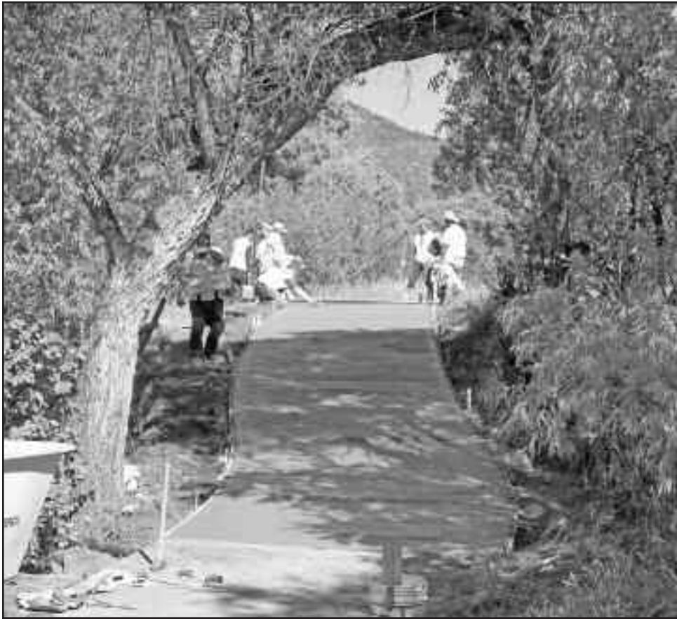
This picture shows concrete being laid on the North Massey Draw Trail. Part of the Trails Master Plan is to convert asphalt paths to concrete. Concrete has a longer life, and it provides a smoother surface for many of our trail users like folks pushing strollers. It also facilitates snow plowing. The change from asphalt to concrete will take place over a 10-year period, and the Master Association is currently in the third year of the project. $100,000 per year is being spent on the conversion. The pathway sections that are in most need are being done first. For questions about the project, contact Master Association Executive Director Chris Pacetti at chrisp@kcranch.org .
