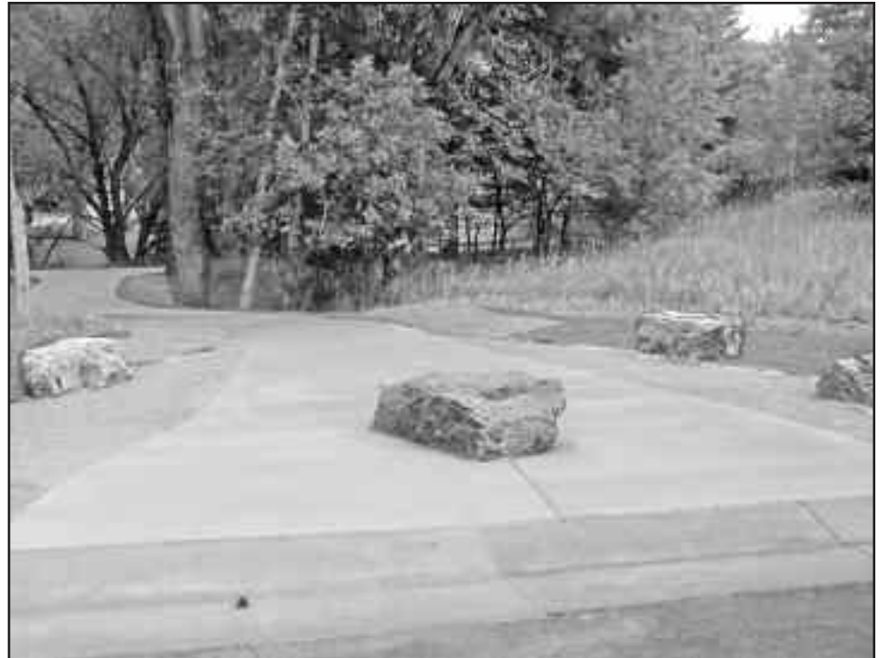
The Dawn Heath Connector Trail was recently paved with a concrete hard surface. The trail connects Dawn Heath Drive to the North Massey Draw Trail. The project cost approximately $9,000 and was completed in July by T2 Construction.
