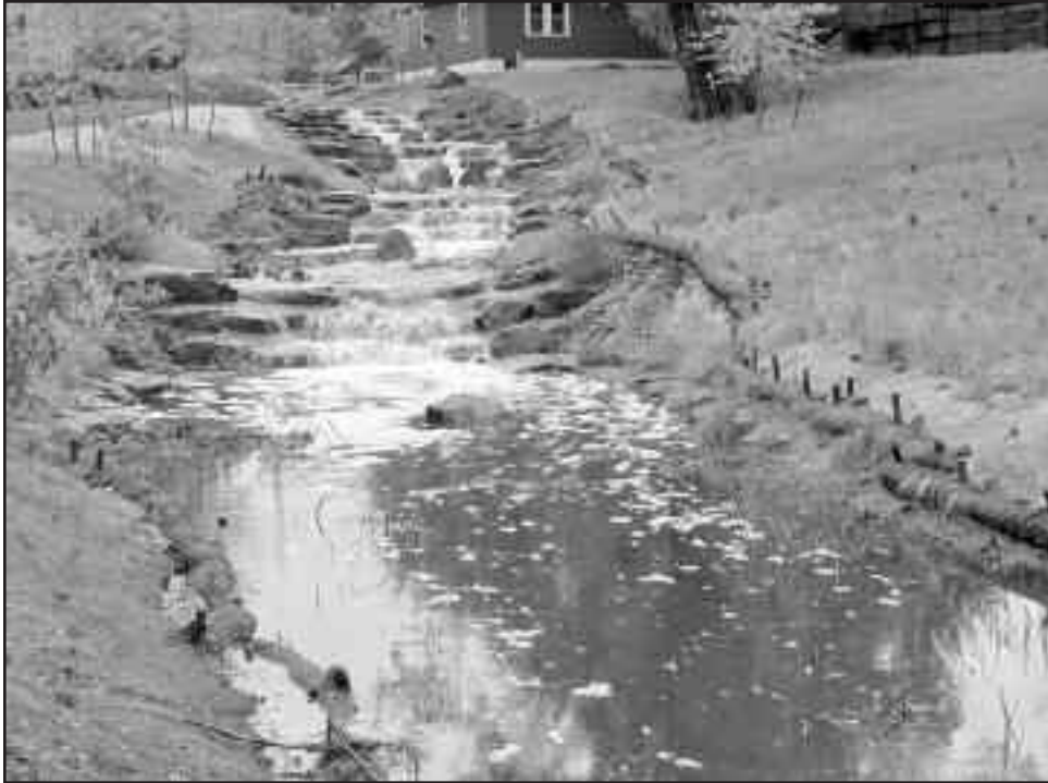
The drainageway improvements adjacent to the Equestrian Center were put to the test during the recent rainstorms, and everything is flowing like it should be. The $380,000 construction project was completed in mid-August. The improvements included removing the undersized culvert and establishing an open channel designed to keep both high and low flows in the same channel.
