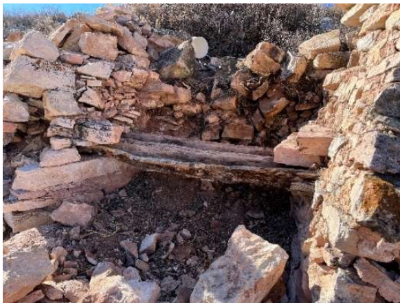
Support beams exposed after the disassembling of the kiln's stoke hole area
