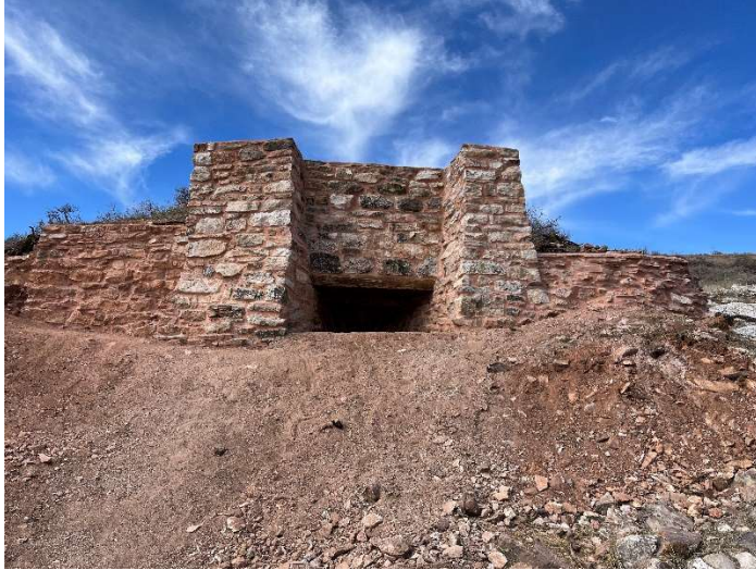
2023 photo after work completion in April. Note the stabilized stone walls adjacent to both sides of the kiln.
